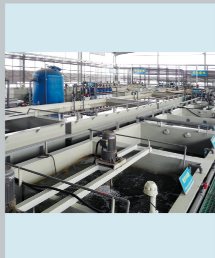
廢水設備 Water treatment
